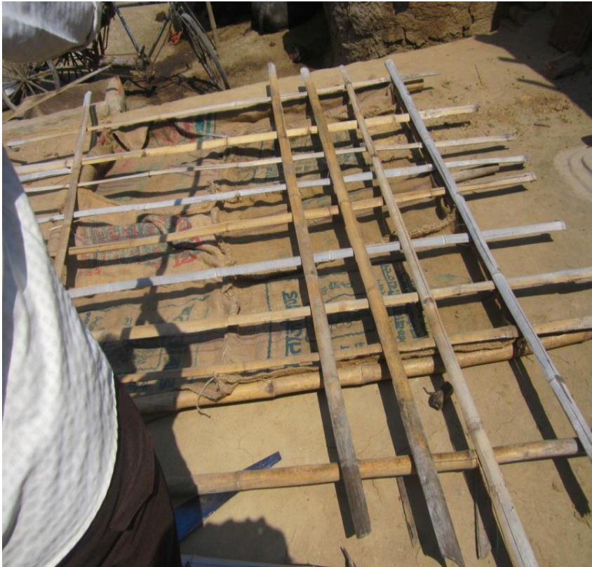
Fabrication of low cost roof using local materials like bamboo and gunny bags
