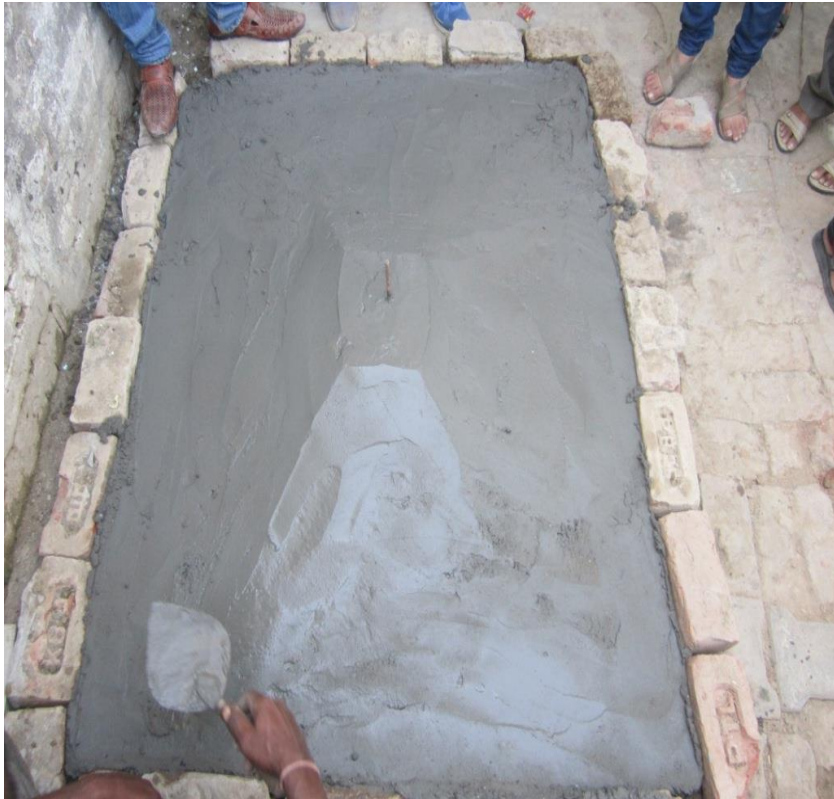
Fabrication of a Ferro-cement Roof top for a Toilet under transfer of technology by Anar Devi Khandelwal Mahila Polytechnic, Mathura at village Chaumuha, Chhatikara near Vrindavan
