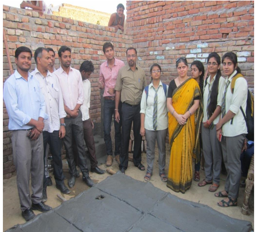
Fabrication of a Gunny Bag/Ferro-cement Roof for a Kitchen under transfer of technology by Anar Devi Khandelwal Mahila Polytechnic, Mathura at village Chaumuha, Chhatikara near Vrindavan
