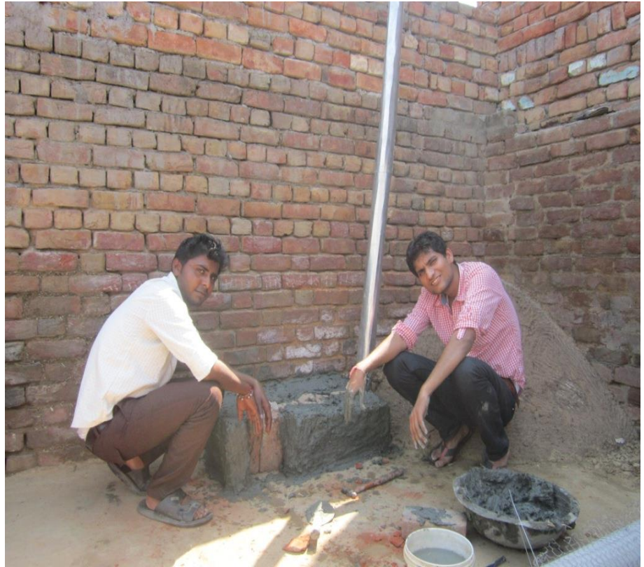
Construction of a smokeless chullah under transfer of technology by Anar Devi Khandelwal Mahila Polytechnic Mathura at village Chaumuha, Chhatikara near Vrindavan
