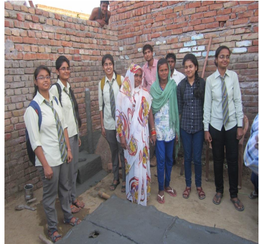
Participation of students and village women in construction of smokeless chullah in village Chaumuha, Chhatikara, near Vrindavan, Mathura
